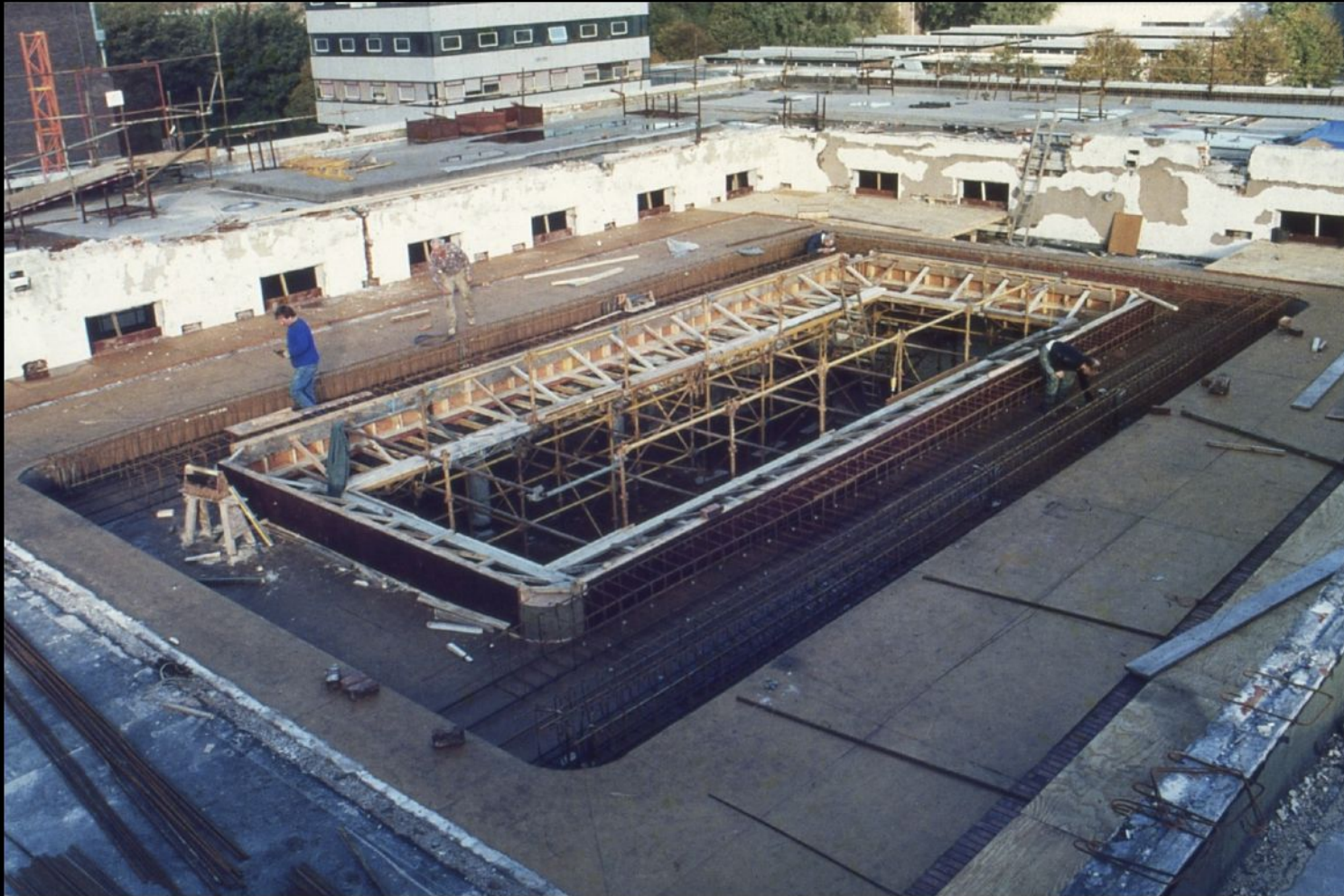
2nd floor slab concrete pour' concrte pump broke and squirted everywhere!
